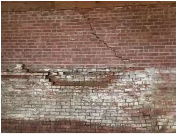
Southeast wall crumbling
